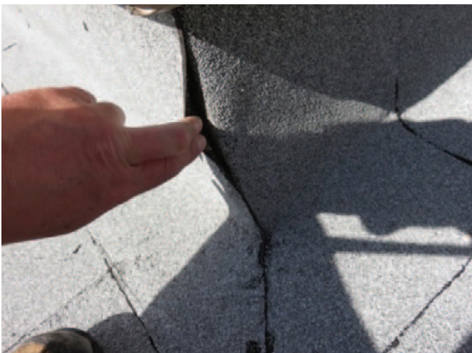
Photograph 2: Drones can provide excellent supplemental information, but some deficiencies are difficult to uncover without a hands-on approach.
