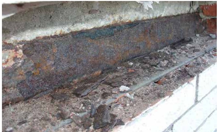
A steel shelf angle exhibiting moisture-related deterioration, resulting in a reduction in load-bearing capacity.
