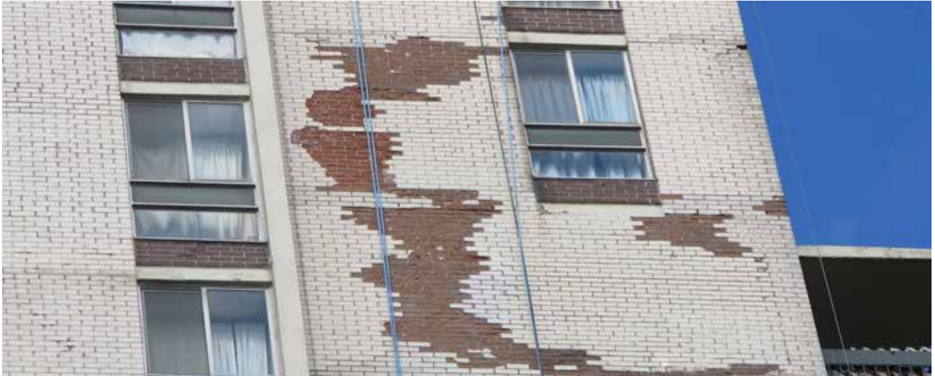
An example of highly deteriorated glazed brick.
