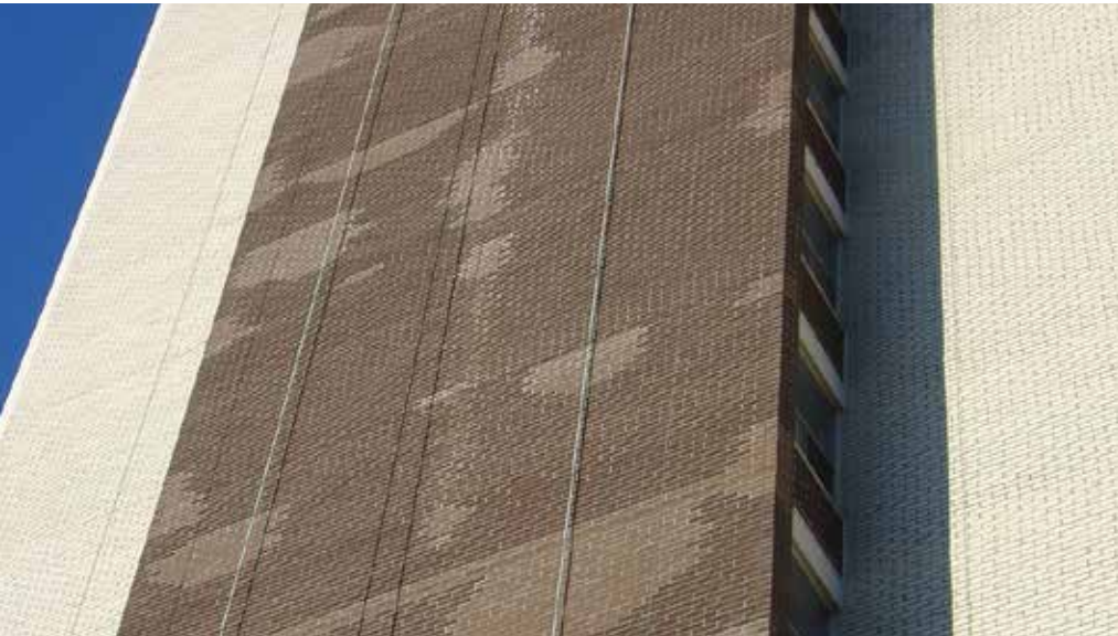
A brick veneer wall exhibiting repairs completed over many years.
